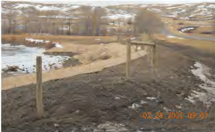
Facing upstream shows the project as it appears completed in late February 2022. Credit: Joe Grosswiler
