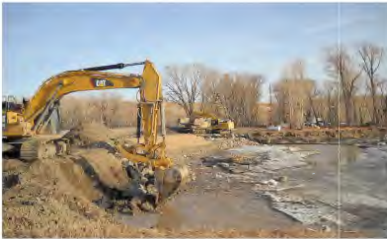
Construction progress on the erosion repair project as of February 2022. Credit: Joe Grosswiler
