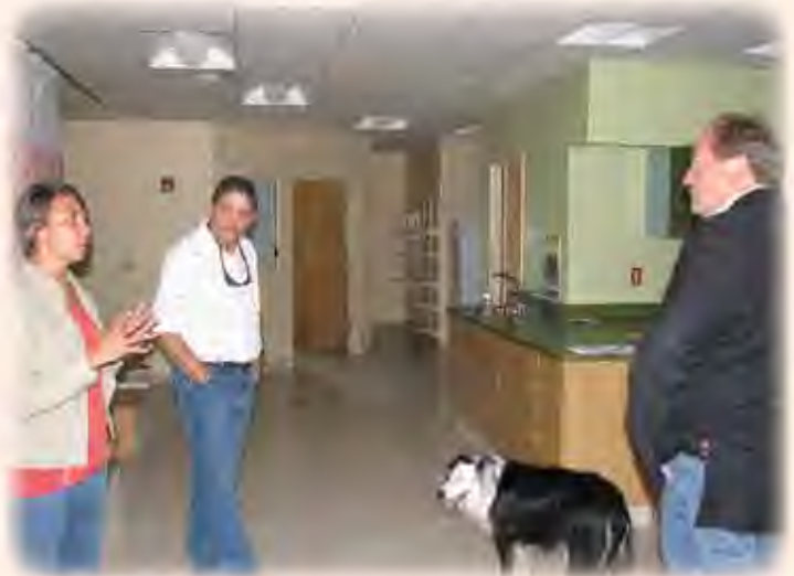
Kim Traversie and Neal Rosette of the Chippewa Cree Tribe brief Governor Schweitzer on the damage to the Rocky Boy's Health Clinic caused by the 2010 flood. (Photo by Lesa Evers)
