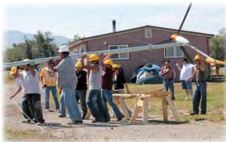
Participants of the Montana State University Great Falls YouthBuild Program installing a wind turbine on the Blackfeet Reservation near Heart Butte (Photo courtesy of Montana State University–Great Falls College of Technology)
