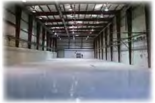
Fort Peck A&S Diversified renovated building (Photo courtesy of Fort Peck Tribes)
