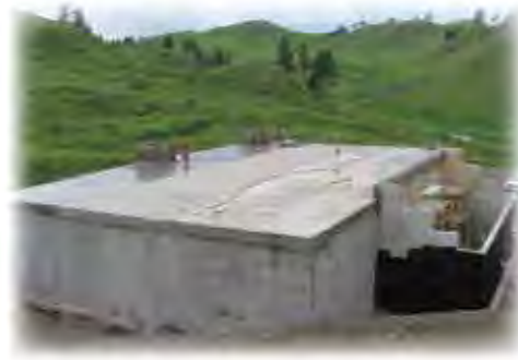
Chippewa Cree Tribe Parker Water Storage Tank (Photo courtesy of the Department of Commerce)
